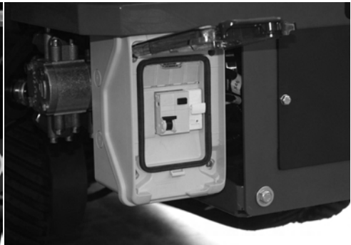
Fig. 142 Main supply switch
