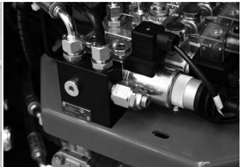
Fig. 10 Ground part pressure relief valve 1
