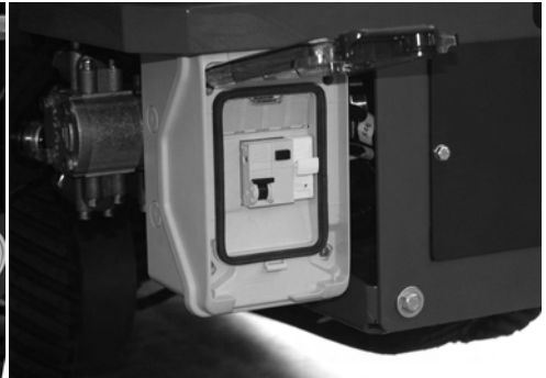
Fig. 82 Main electric switch
